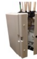
Property node The interface between Property owner and Stokab
