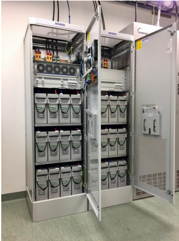
Fig. 1. The time node sites have uninterruptible power supply (UPS) such as battery and diesel generators. In addition, the time keeping equipment in the node has 24 VDC battery for another three days.
